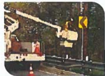
Electric and Existing Pole
