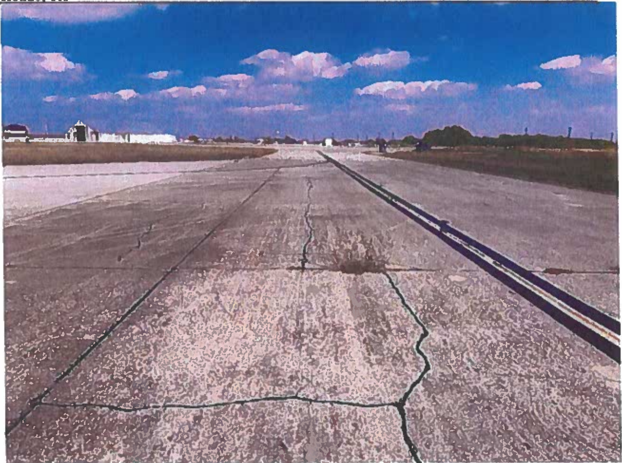
Figure 5 - Exposed vegetation looking northeast at intersection of Taxiway A and E (Site Visit 10/24/22)
