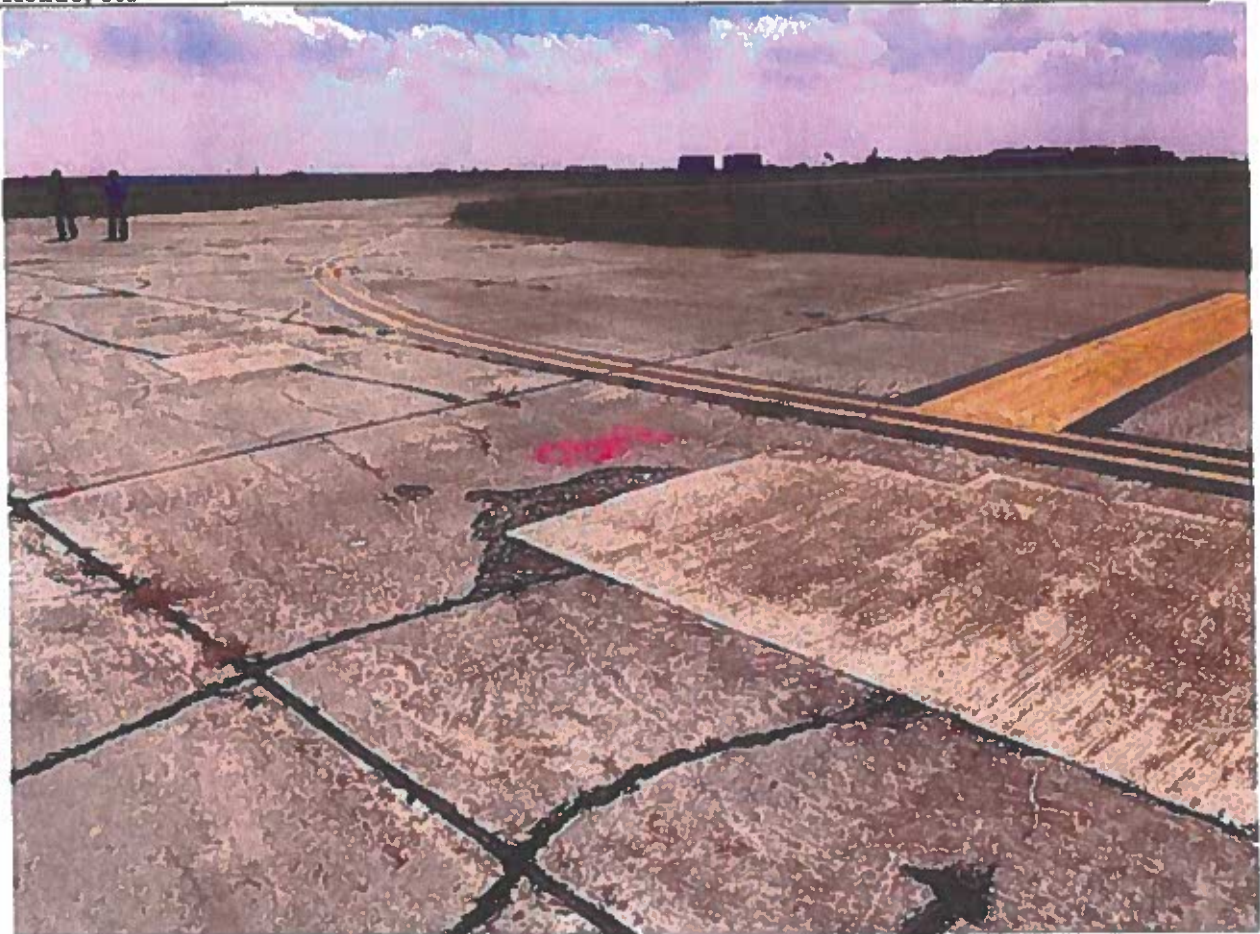
Figure 3 - Severe distressed concrete near B-1 with patch work and exposed aggregate. (Site Visit 10/24/22)
